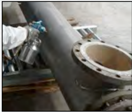
Insulation & Corrosion Control Guadalajara, Mexico
