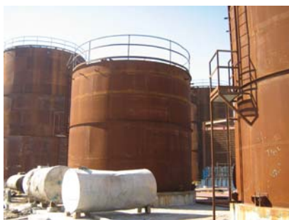
Methanol tanks suffered from corrosion and vaporization of liquid due to hot climate.
