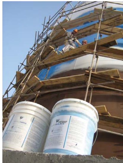
Nansulate® Top Coat, which is a white, semi-gloss was tinted blue per customer's needs and used as the final overcoat
