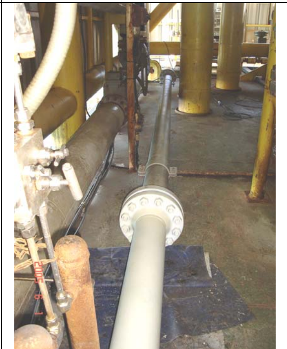
Transition of the final section to the middle one with the work done
