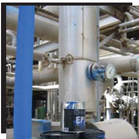
Pipelines and Tanks
