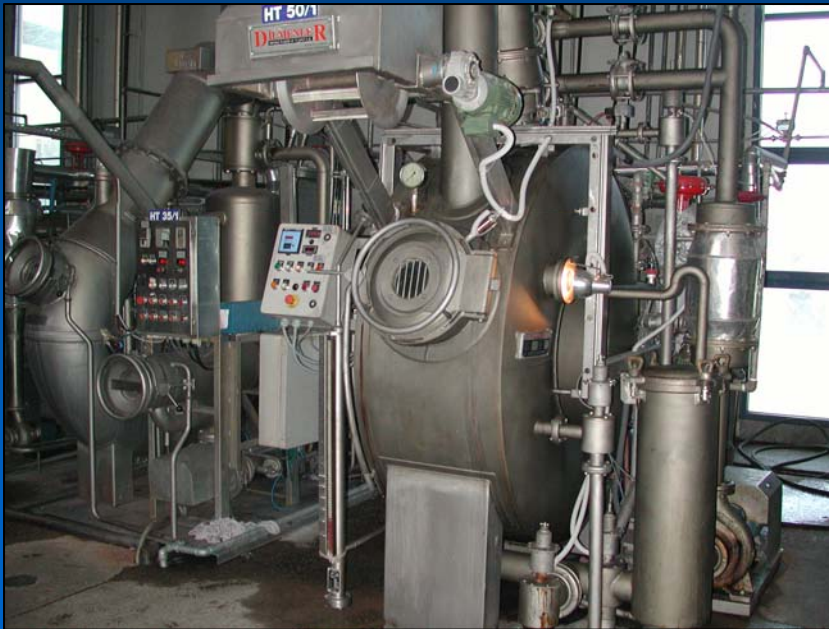
Heat Exchanger insulated with Nansulate®
